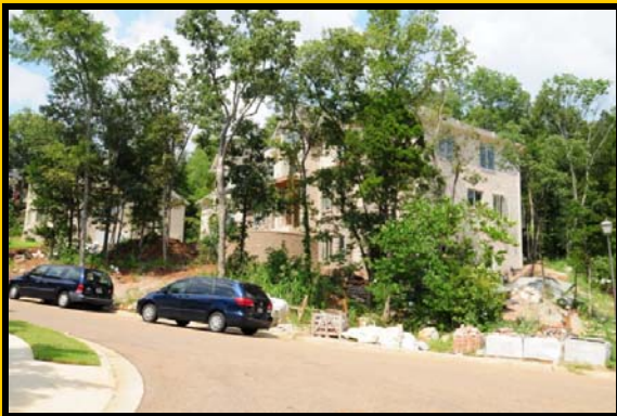
Srilatha and Vijay Jampala resumed work on their Springhouse Lot 57 home and rapid progress is being made.
